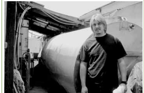
Josh Fraka, Insectary Technician and Carpenter working on installation of our solar hot water storage tank.
